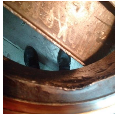
Local damage on topland ring
