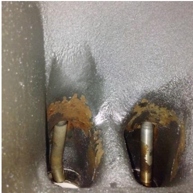
Damaged valves stems, air intake side
